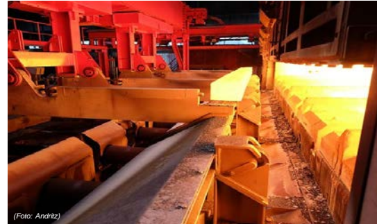
Hubherdofenanlage In Witten (DE) DEW (2020)
